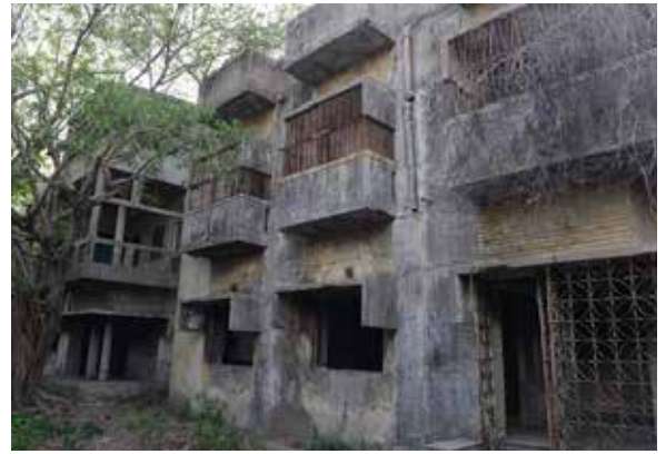
Abandoned and damaged Buildings owned by Muslims in in the Gulberg Society, Ahmedabad. 69 Muslims sheltering in this residential complex were murdered on during the anti-Muslim pogrom of 2002. Photo: SAM PANTHAKY/AFP via Getty Images
